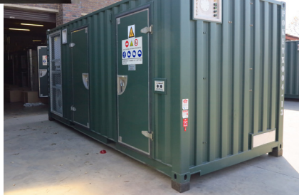
Picture 2: Containerised shelter
